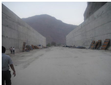
Kryton's waterproofing products were used to treat tens of thousands of square meters of concrete at the dam.
