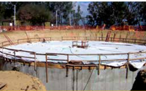
TreePeople Center Underground Cistern, Los Angeles, California, USA
