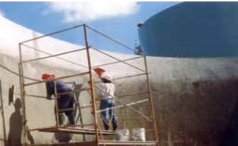
Annacis Island Wastewater Treatment Plant, Vancouver, British Columbia, Canada
